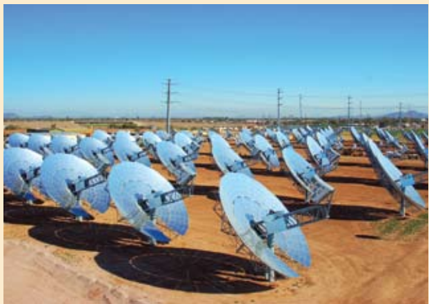
Maricopa Solar in Peoria is a result of a partnership between Salt River Project (SRP) and Tessera Solar. Photo: Tessera Solar
