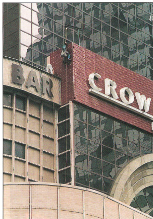
Repairing and maintaining Times Square signs is an ongoing task that can take workers from street level to skyscraping heights. (Photo by David Rinella.)
